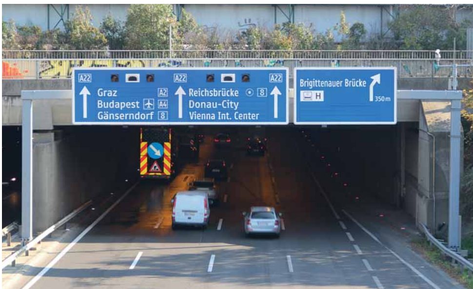
Gantry fitted with prism-type variable message signs
